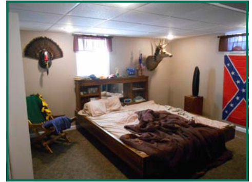
Basement Non-Conforming Bedroom
