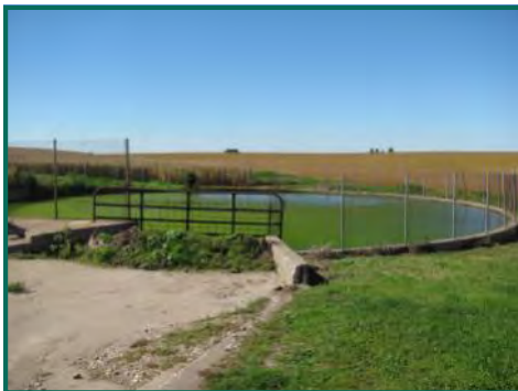
Concrete Manure Pit
