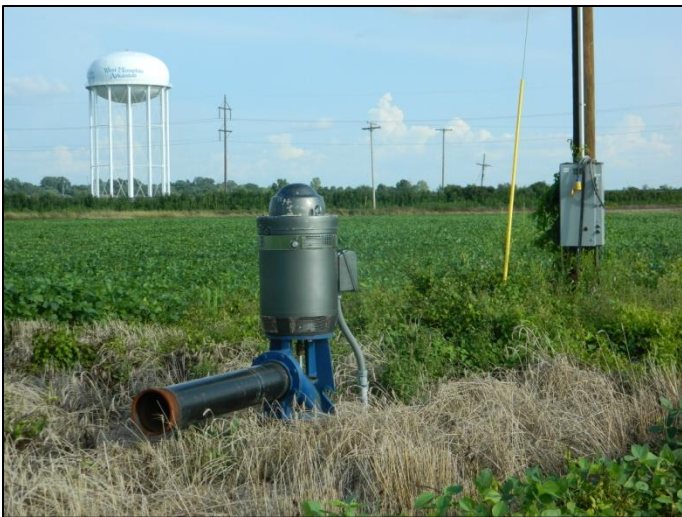
Well, Motor, and Panel to Transfer
