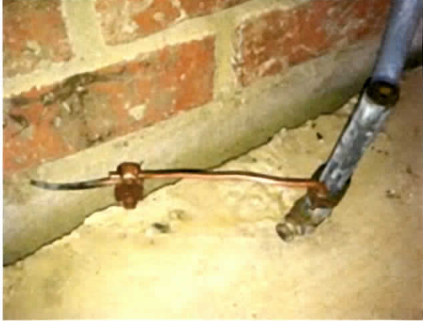
redid ground to house, located on carport
