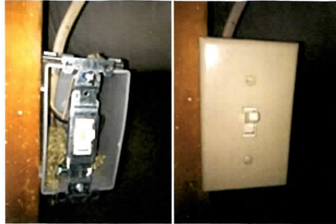
uncovered switch in attic - covered with plate
