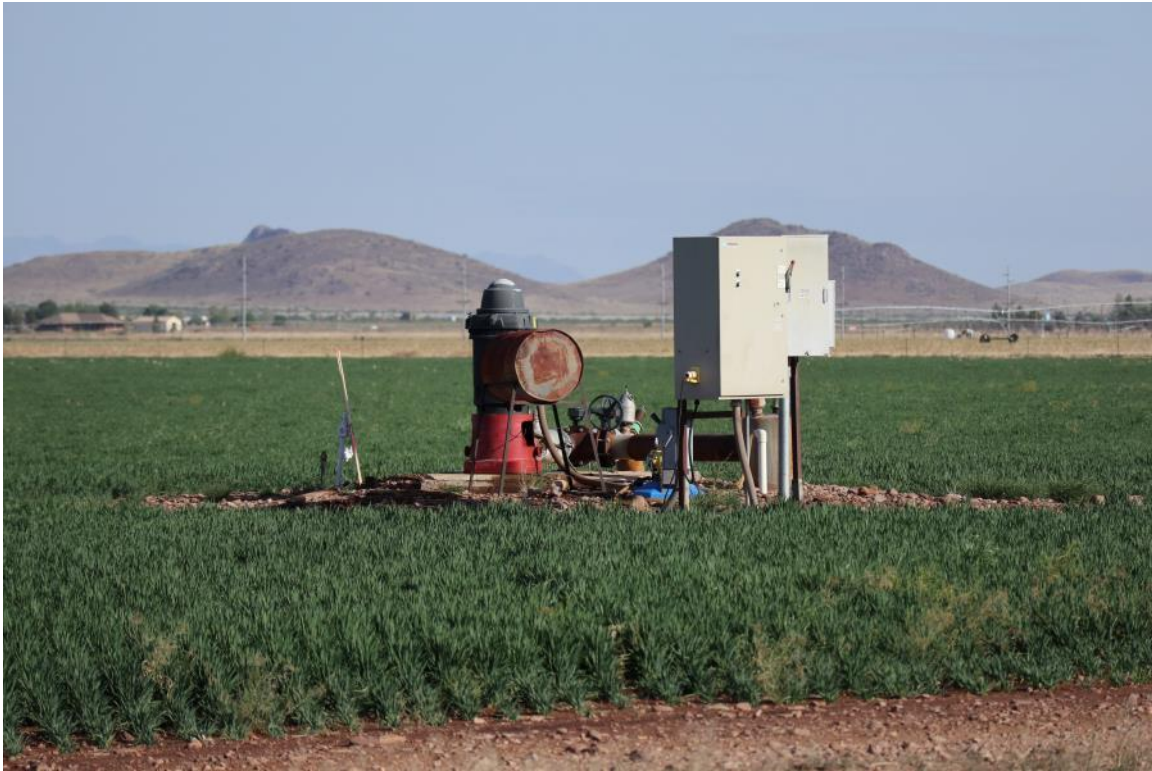
Well no. 24, 600' deep, 125 HP, 700 GPM
