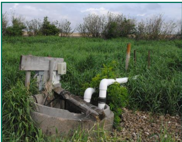
Sump Pump - East side of Farm
