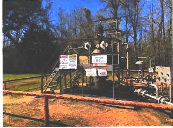
VIEW OF TYPICAL GAS WELL
