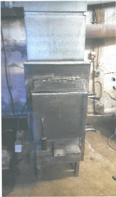
Wood burning furnace in the central system
