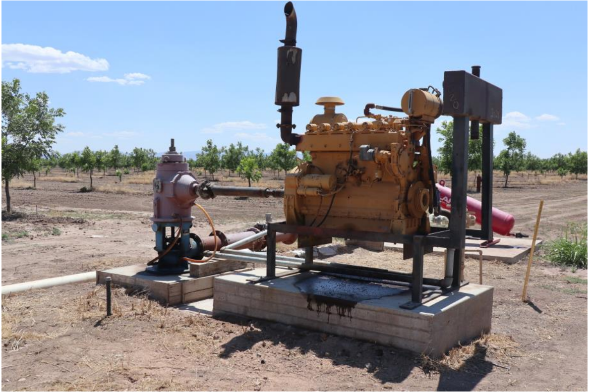
Natural gas driven irrigation pump
