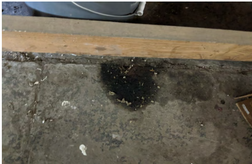
Photo 27. View of minor floor staining.
