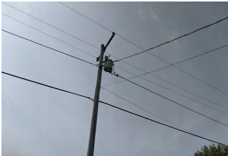
Photo 37. View of pole-mounted transformer in the vicinity of the subject site.
