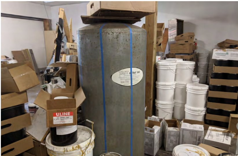
Photo 23. View of empty air float tank.
