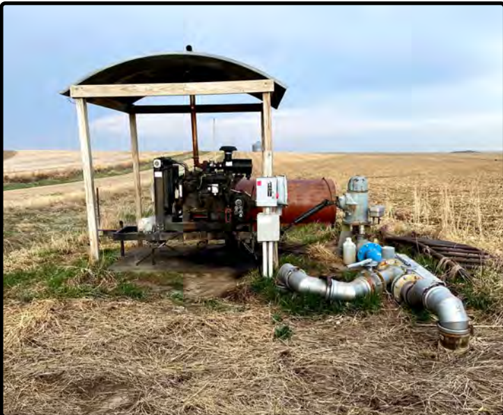
Parcel 2 - Well, Motor & Diesel Tank
