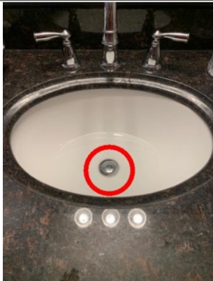
Left side bathroom sink stopper does not hold water.
