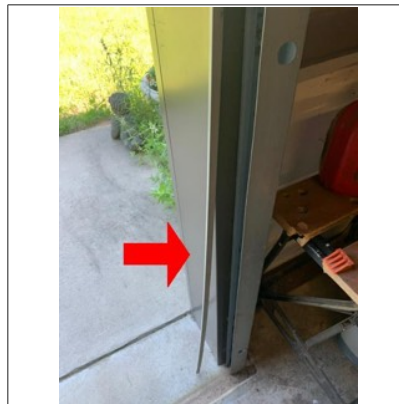
Loose weather stripping on overhead door.
