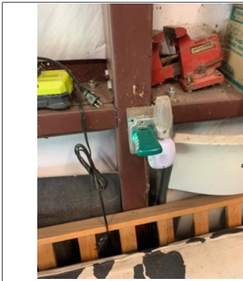
Shop and laundry room outlets are not GFCI protected.
