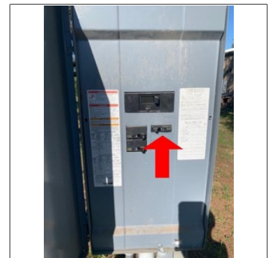
Not all breakers are labeled at service panel.
