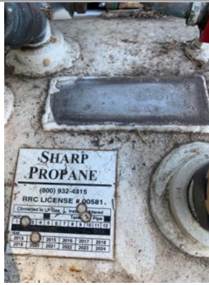
Label on the propane tank.
