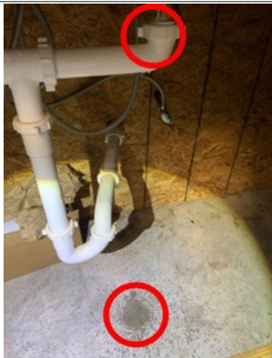
Waste pipe is leaking under shop sink.
