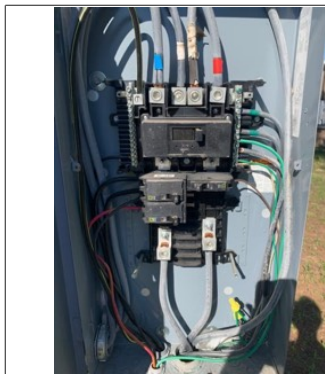
Inside view of the service panel.
