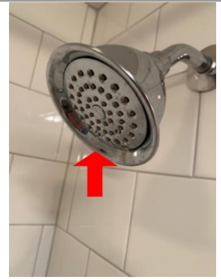
Left side shower is leaking.
