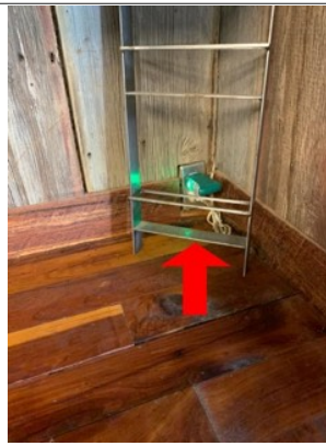
Sink area outlet in shop is not GFCI protected.
