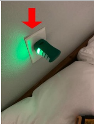
Outlet loose in the wall in left loft.
