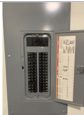
The sub-panel is in the laundry room. Not all breakers are labeled.
