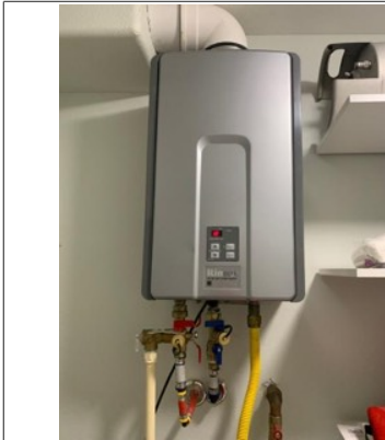
The tankless water heater is in the laundry room.
