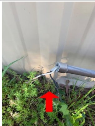
Abandoned wires in conduit at the rear of the building.
