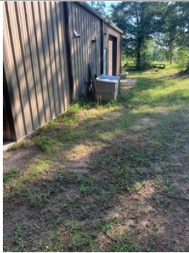
No slope away from building on the right side.
