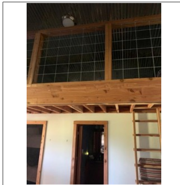
No emergency exit for lofts.
