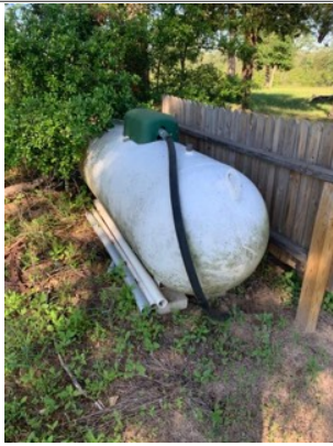
Propane tank to the right of the building.
