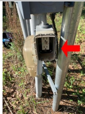
Outlet under the service panel needs to be better secured.
