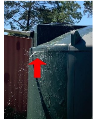
Overflow at storage tank.
