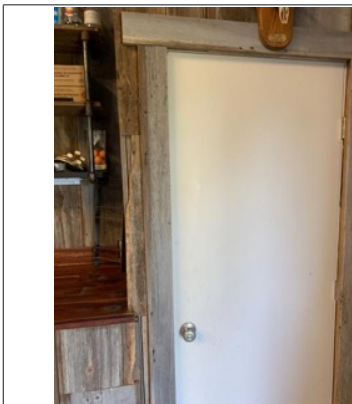
Closet door in shop needs adjustment/trimming.
