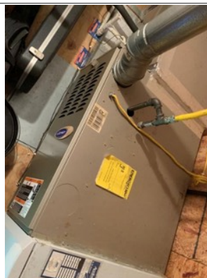
The furnace is in the attic above the laundry room.
