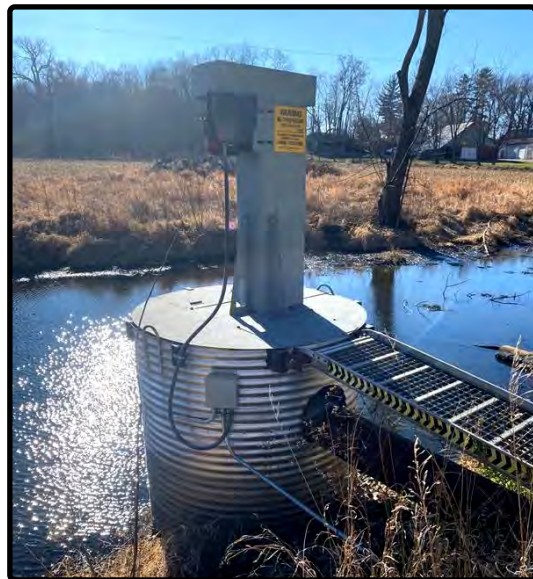
West Lift Pump
