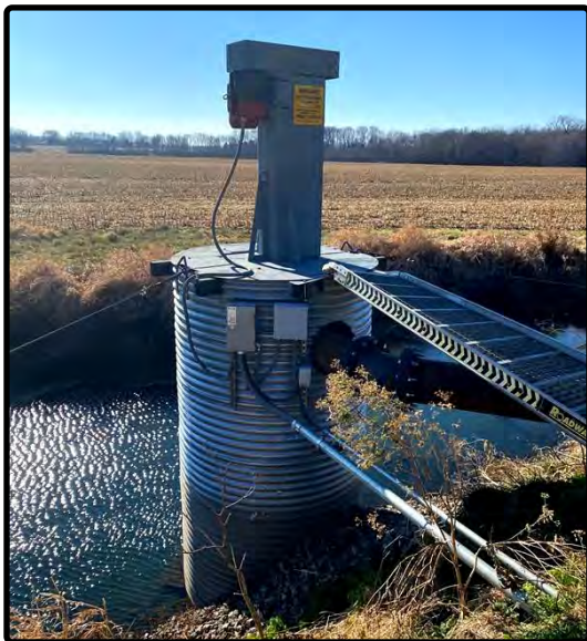
East Lift Pump
