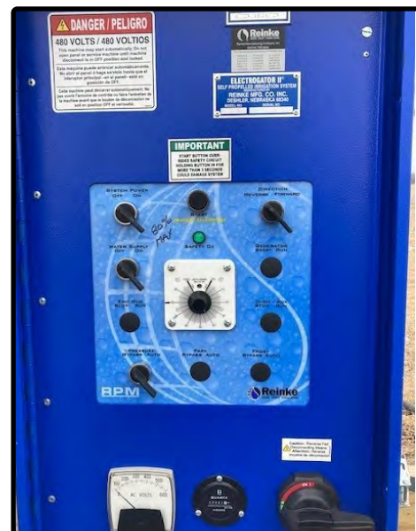
Panel 2 on North Tower
