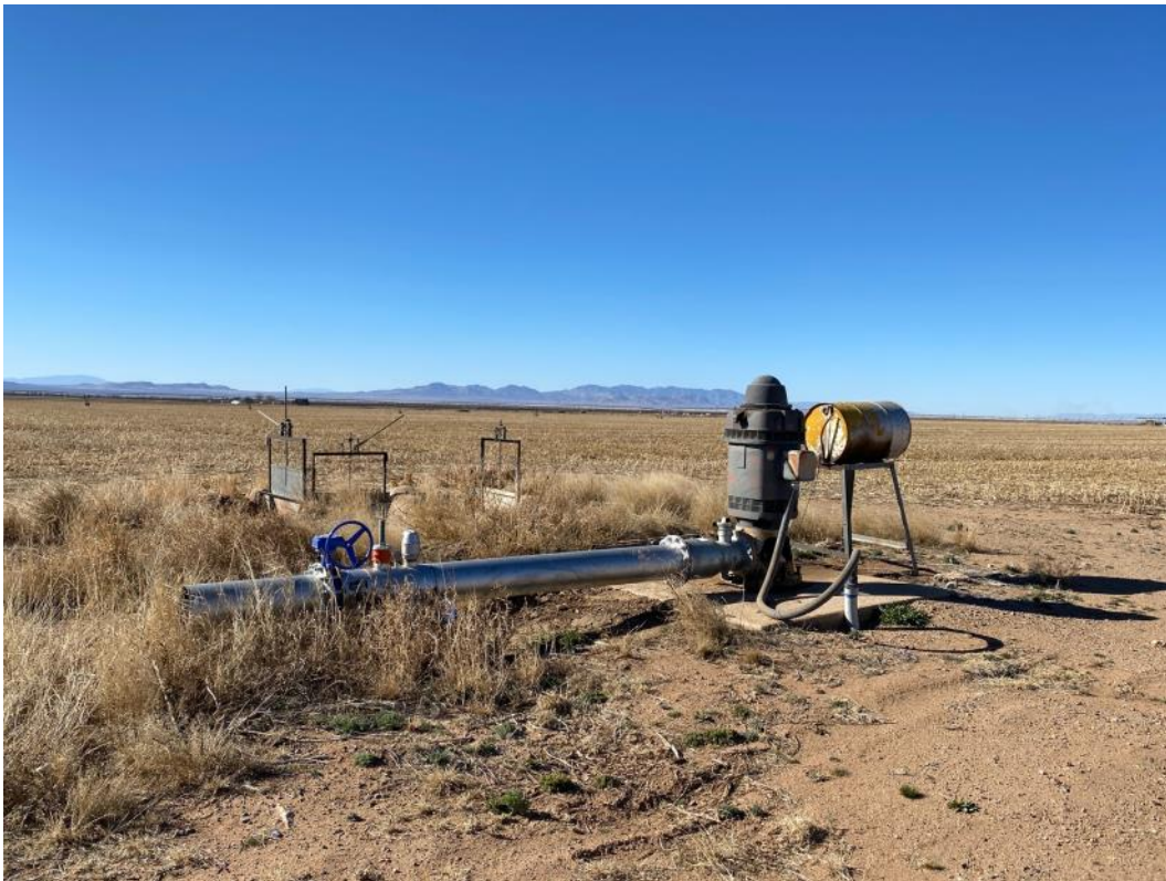
Irrigation well, 610' deep, 200 HP, Approx. 650 GPM
