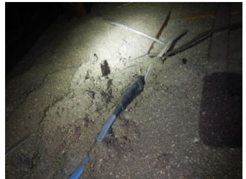
wire splice not in junction box
