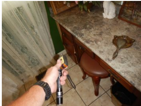
Bathroom outlet(s) not GFCI protected
