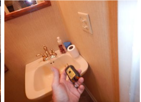
Bathroom outlet(s) not GFCI protected
