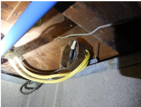
Junction box missing cover
