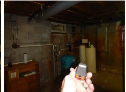
unfinished basement outlet(s) not GFCI protected
