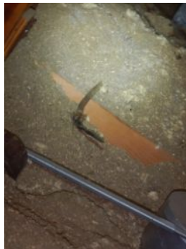
Unterminated wires should be properly terminated inside junction box or removed
