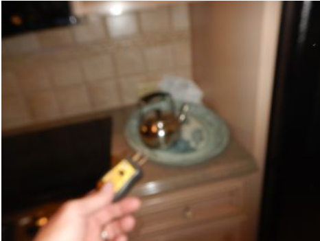
outlets above kitchen counters are not GFCI protected
