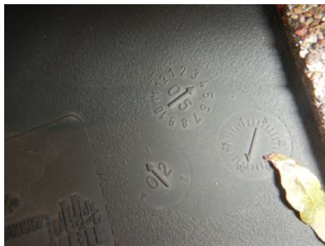
penetration boot is dated 2005
