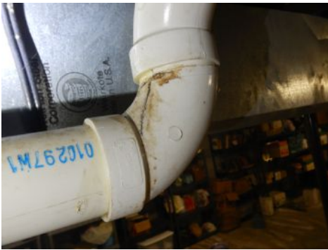
signs of (past?) leaking
