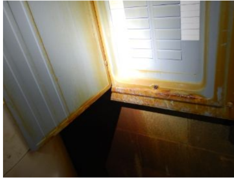
rust/ iron stains from (assumed) past leak by water softener
