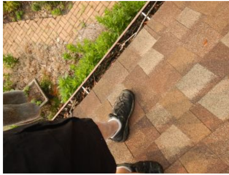
soft spots in roof by eaves (front of house)
