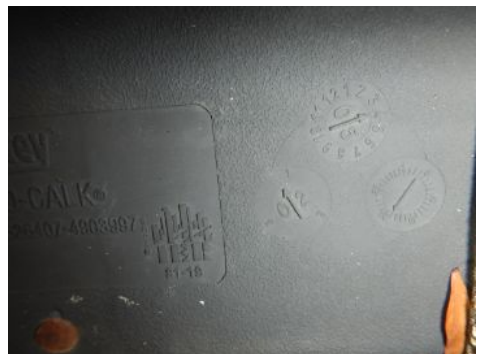
penetration boot is dated 2002
