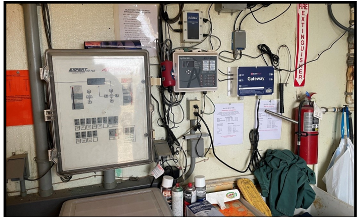
Ventilation Controller & Alarm System
