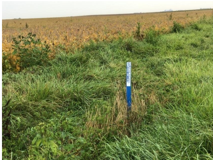
Water valve along E 8000 North Rd
