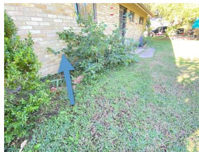
Foliage in contact with structure- rear left
