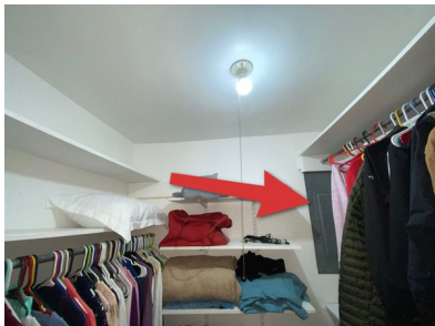
Main electric panel installed in master bedroom closet
