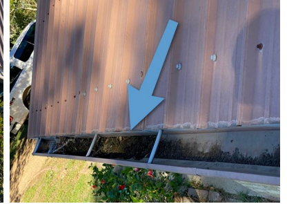
Debris in gutters - front left
