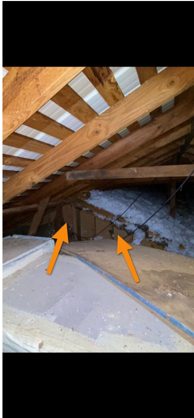
Knee wall insulation missing or out of position
