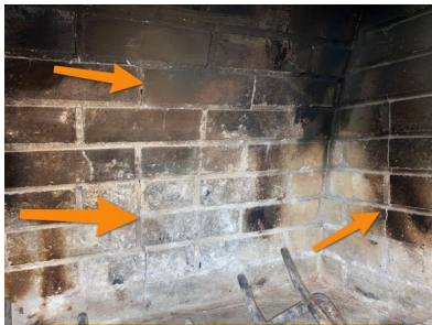
Cracked bricks and mortar joints at firewall
