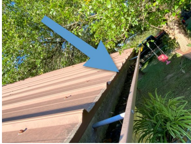
Debris in gutters - rear left
