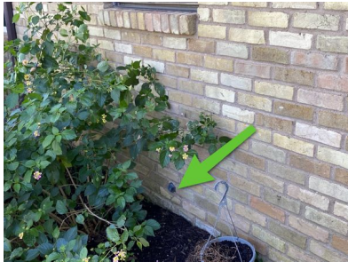
Drain cleanout in exterior wall behind kitchen sink
