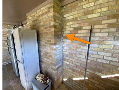
Cracked mortar at corners of chimney/fireplace
