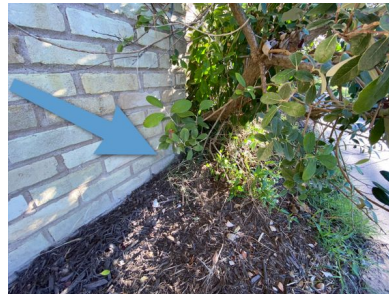
High soil - bed near front door
