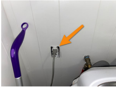
Missing cover plate at washing machine receptacle
