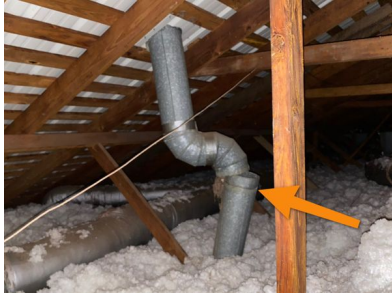
Range hood exhaust duct separated
