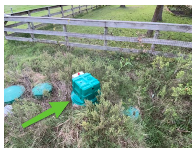
2nd tank - aerator chamber
