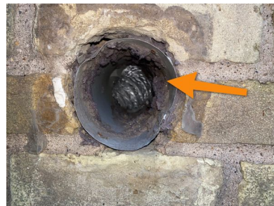
No damper at dryer exhaust
