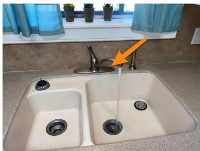
Kitchen faucet is loose at countertop
