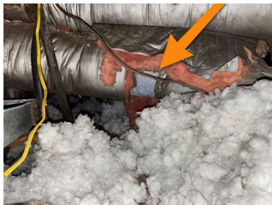
Damaged AC duct insulation
