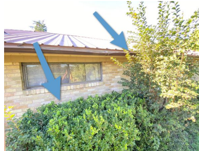
Foliage in contact with structure - rear middle
