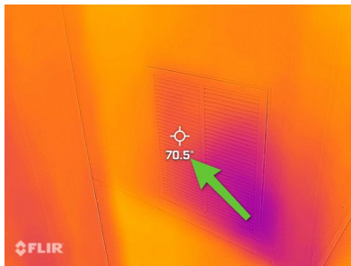
Cooling temperature reading at return
