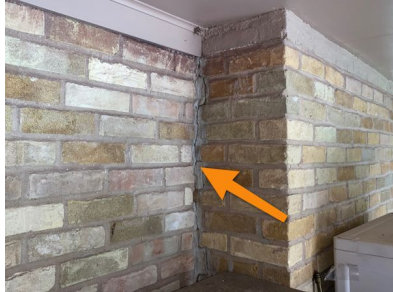
Cracked mortar at corners of chimney/fireplace
