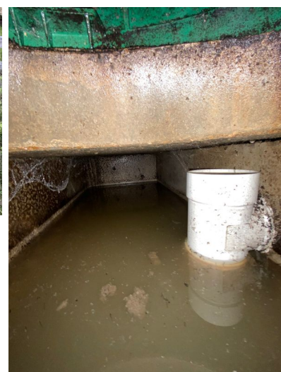
2nd tank - clarifier chamber
