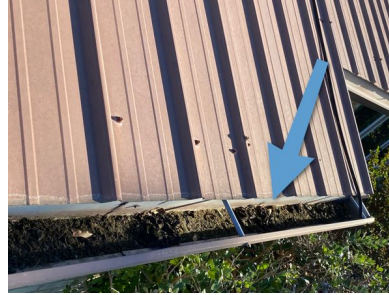
Debris in gutters - front left
