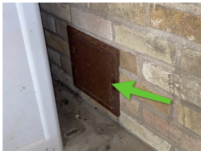
Ash cleanout located on exterior behind fireplace
