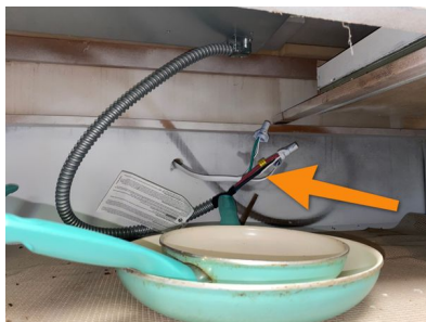
Open splices at cooktop wiring
