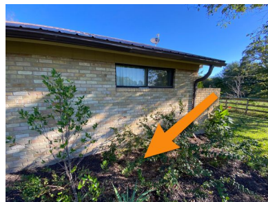
Large depression below gutter leak at front right
