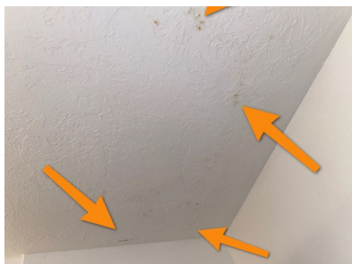
Minor staining, paint flaking above shower
