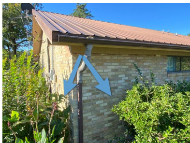
Foliage in contact with structure- right side and rear left
