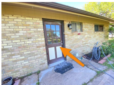
Rear exterior door needs adjustment
