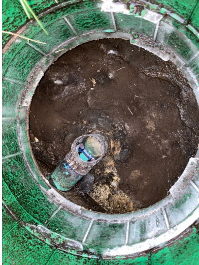
Excessive solids in first tank
