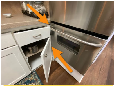
Oven door handle restricts cabinet door and drawer opening
