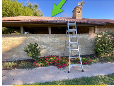
Roof deflection/dip above carport
