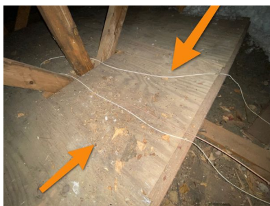
Small section of attic flooring above carport is too thin
