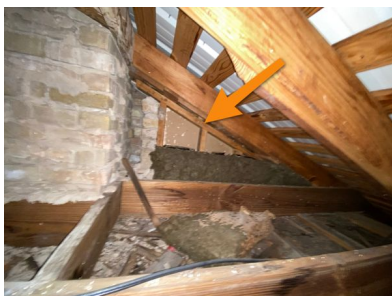
Insulation missing from kneewall
