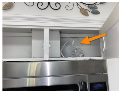
Open splices at microwave wiring
