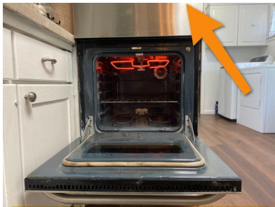
Upper oven producing inadequate heat
