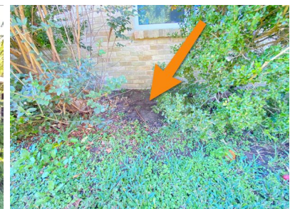
Excess moisture in soil below gutter seam leak
