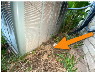
High soil at back of AC condenser
