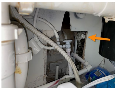
Back wall of kitchen sink cabinet is open to exterior wall cavity
