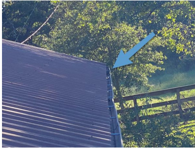
Debris in gutters - front right
