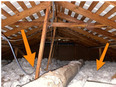
Attic insulation depth insufficient
