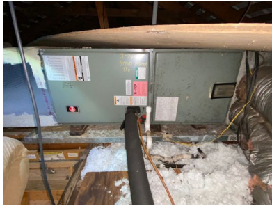
Air handler (furnace)
