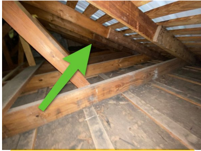
Minor rafter sag causing deflection in roof
