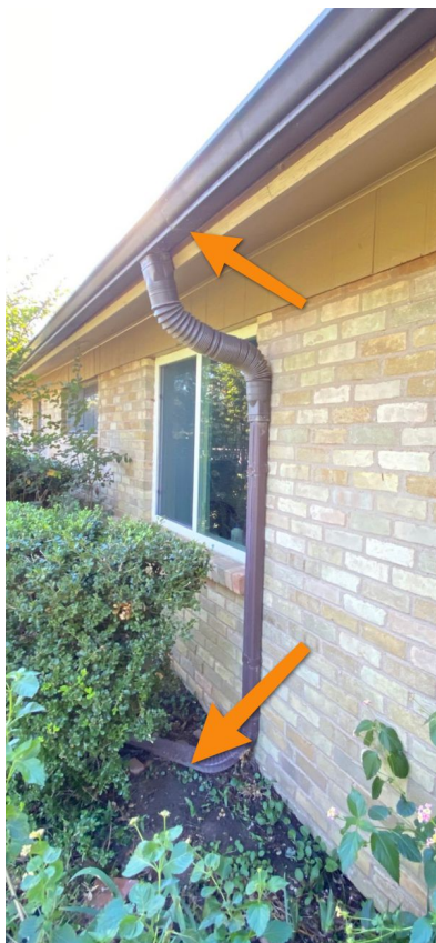
Rear middle - gutter seam leaking
