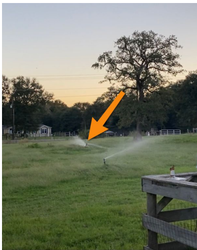
Leak at spray head
