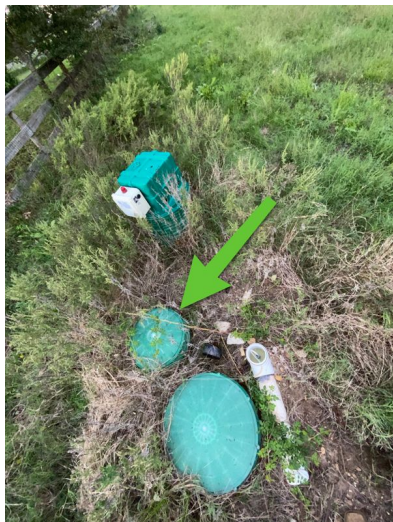
2nd tank - clarifier chamber
