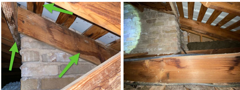
Water stains in attic near chimney
