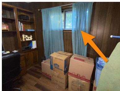
Window in study not suitable for emergency egress
