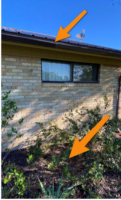
Front right - gutter seam leaking, excess moisture and erosion at soil below
