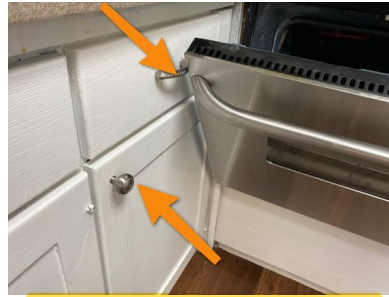
Oven door contacts cabinet hardware when opened
