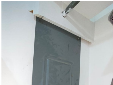
Screws at top of panel obstructed by shelf support
