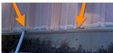
Minor rust at bottom edges of roof
