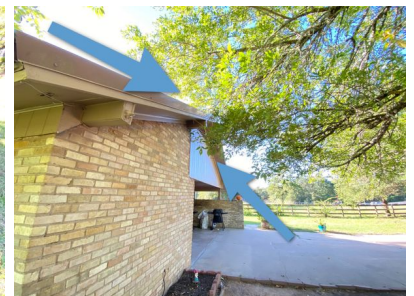
Foliage in contact with structure - left side
