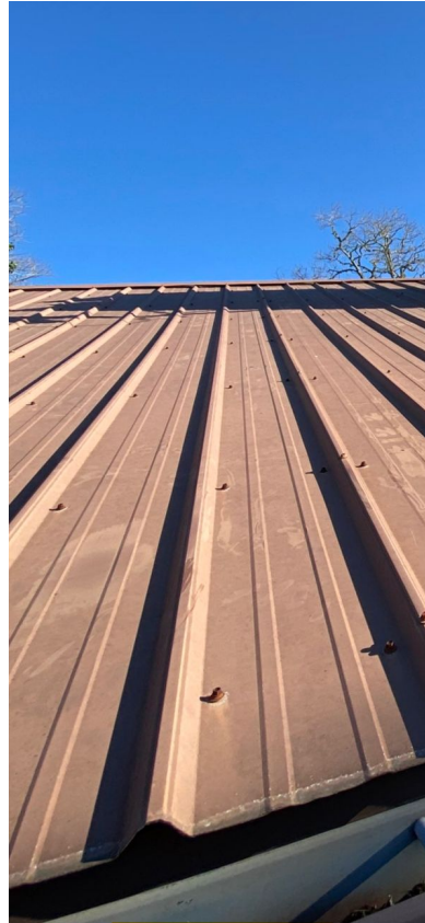
Rusted roof fasteners
