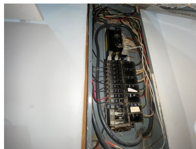
Main electric panel
