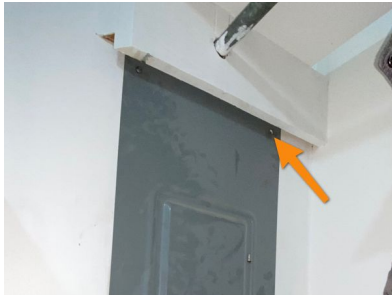
Missing screw at main electric panel
