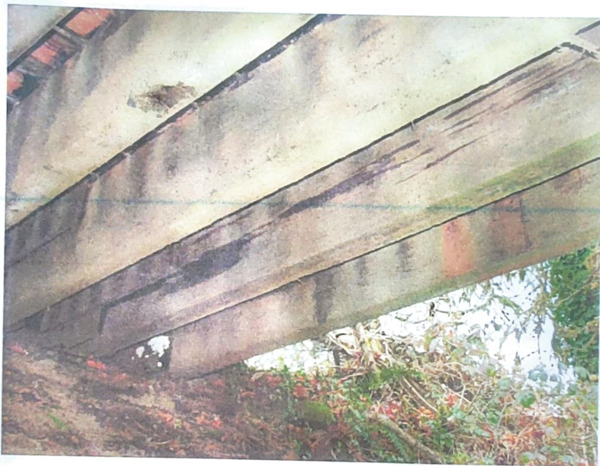
Photo 2. The second stringer from the right has an area of decayed wood where the wood is darker. This decay will continue to propagate. Not also the timber side members attached to the second and third stringer from the right.
