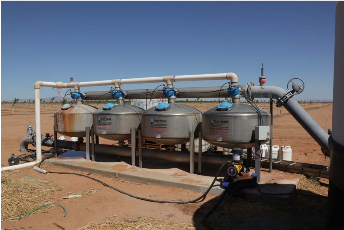
Drip irrigation filtration system
