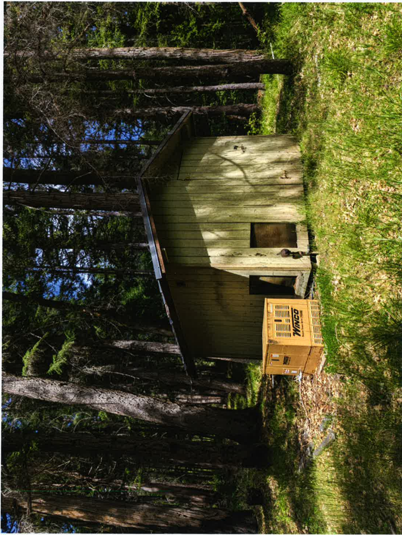
Pump house with generator
