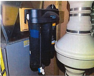
House Reverse Osmosis System
