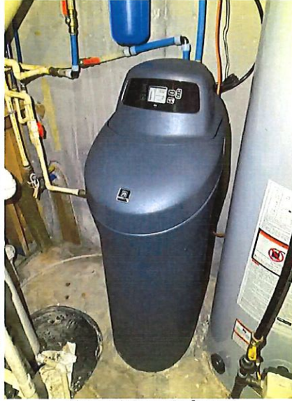
House Water Softener
