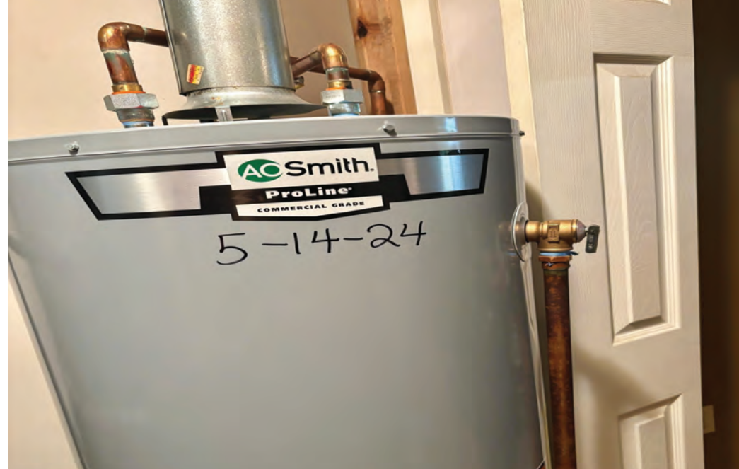
New water heater
