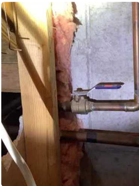
Main shut off above pressure tank
