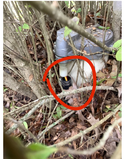
Well conduit pulled apart.
