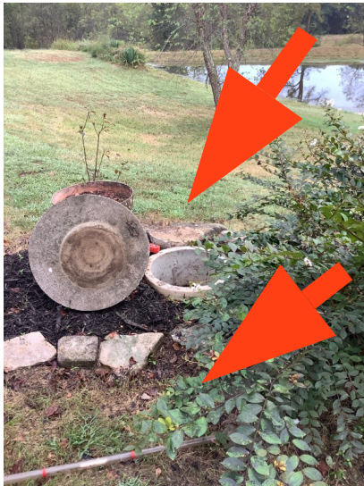
Tank missing inspection ports.
