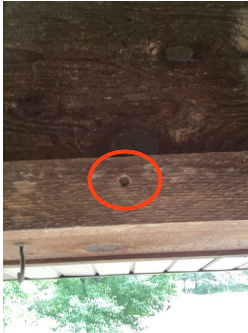
Front porch carpenter bee holes.
