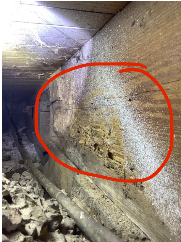
Basement exterior stairwell joist looking towards kitchen termite damage.
