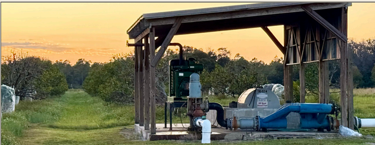
12" well with new power unit.
